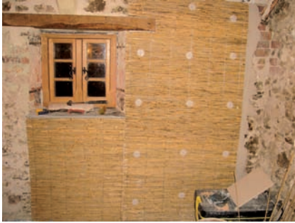
New lintel and bespoke window fitted – reed insulation being fitted with lime mortar backing
