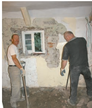
Graham and Bob preparing the room by removing the cement plaster and flooring – the lintel over the window can now be seen to be failing
